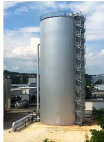
District heating, Ulm Germany
