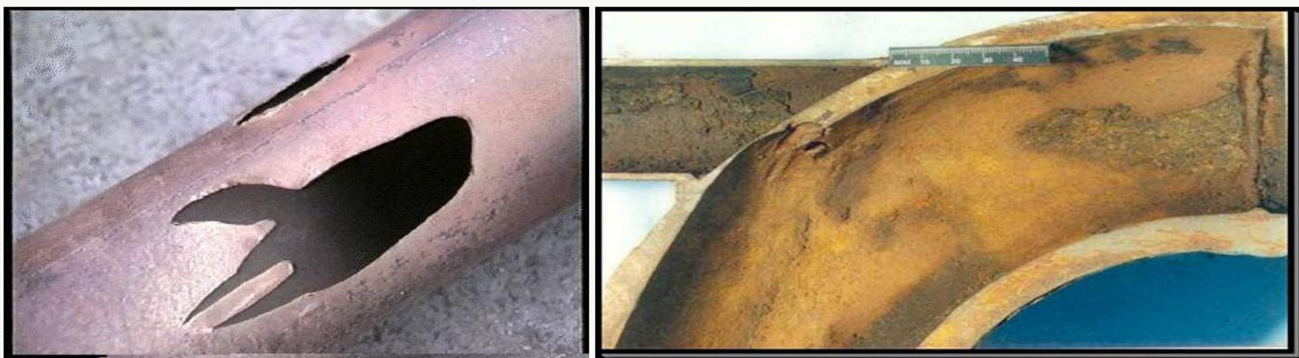
Figure 4: Erosive wear damages of conveying pipelines of bulk materials
