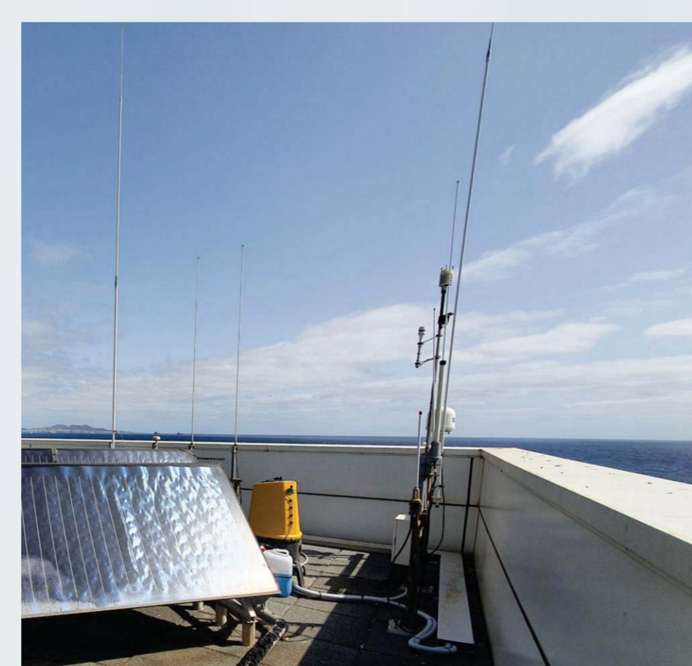
Figure 2. Site instrumentation, LIDAR (yellow equipment) and air quality station (white one)
