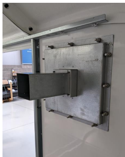
Figure 11: LEV duct with exhaust fan installed on the side of the trailer.
